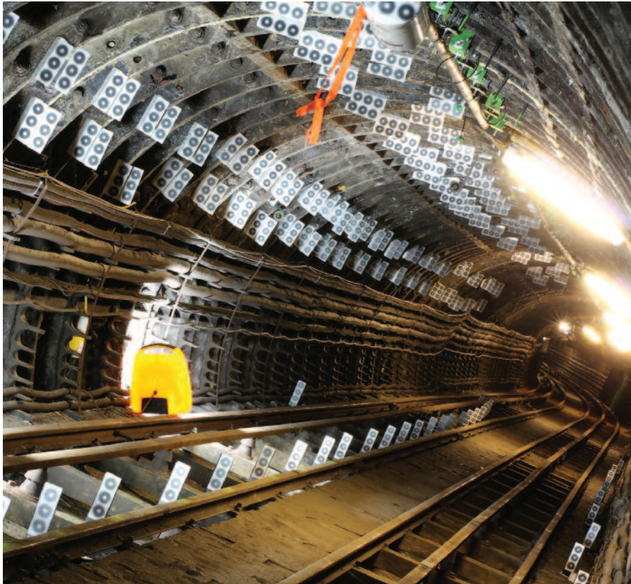
Smart tunnel with monitoring devices
